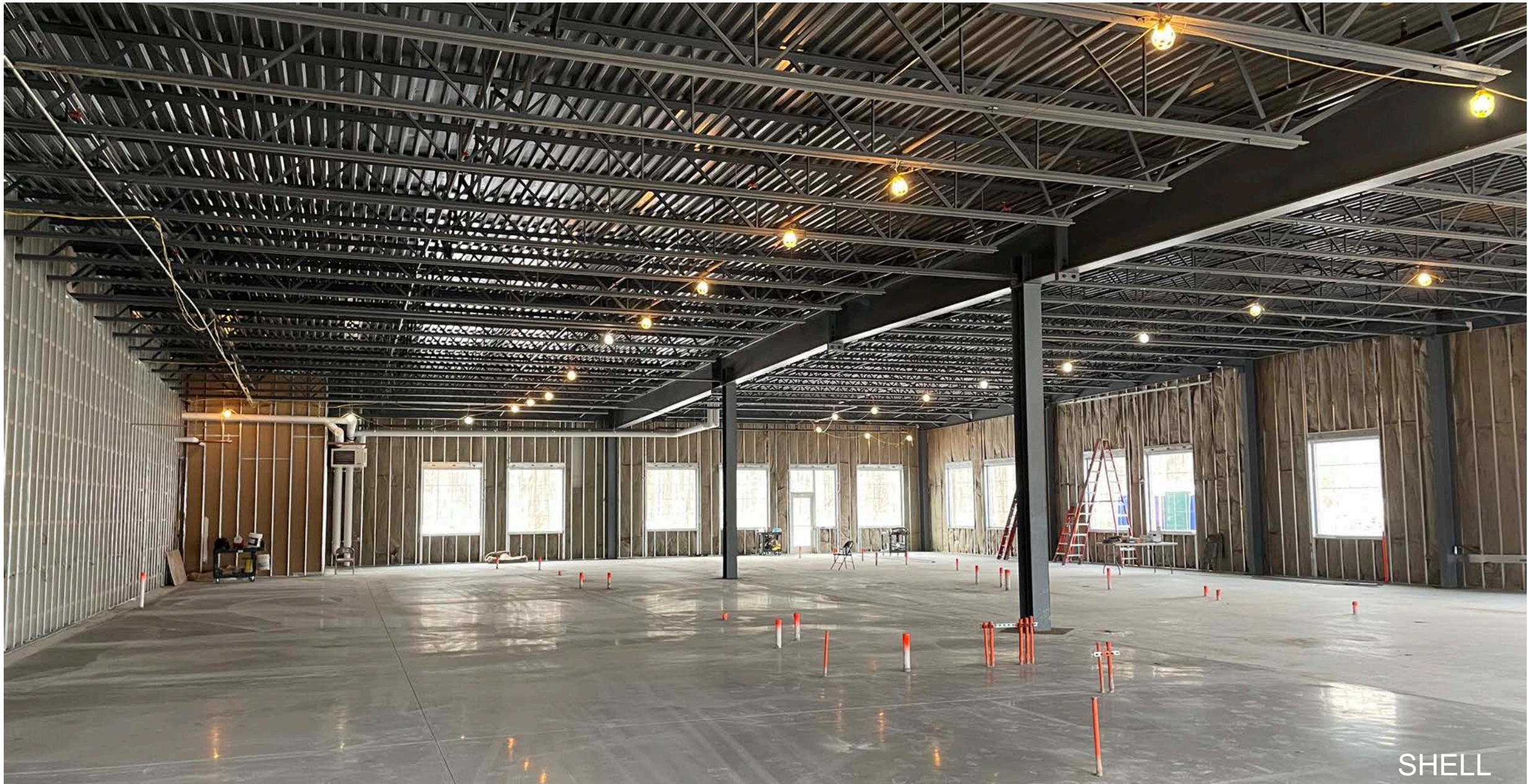
The shell of the project was in design while tenant improvement design was being finalized. Design challenges were resolved through coordination with the contractor. These included floor penetrations set prior to concrete being poured, changing size of the shared mechanical room, door/window opening locations, and the demising wall shifting location during the design phase.
